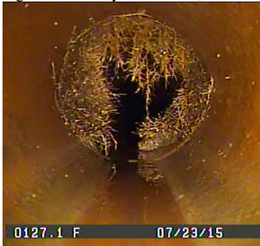
Figure 5: Sanitary Sewer Line, Tree Root Intrusion
