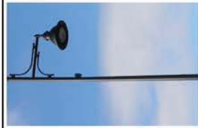
Intersection/Boulevard Lighting Without Banners
