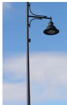
Intersection/Boulevard Lighting Without Banners
